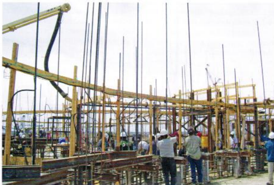
The 24-hour operation meant rebar was continuously tied on as the forms rose.
