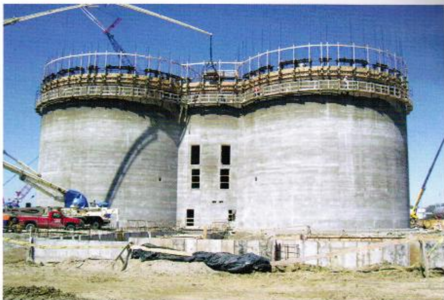
Twin 146-foot tall silos were slipformed continuously, with a core wall joining them together.
