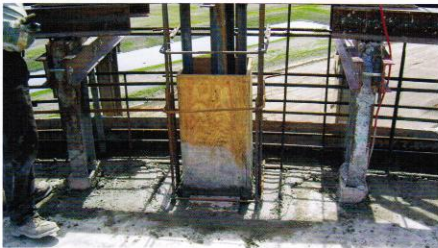
The concrete was deposited from the placer onto the floor of the climbing form. Laborers pushed the concrete into the form to maintain the correct volume.
